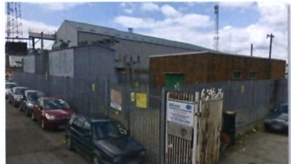
Figure 06: Electrical sub-station [Google Street View]
